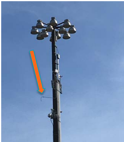
T18 Antenna on Light Pole
