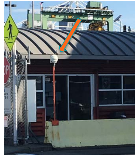
T18 "Exciter" at Gate 4
